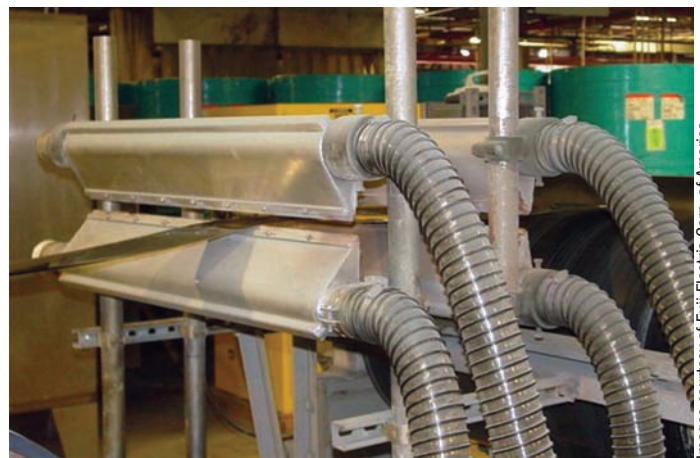
Close-up of air knives showing flexible hoses leading from blower plenum.
