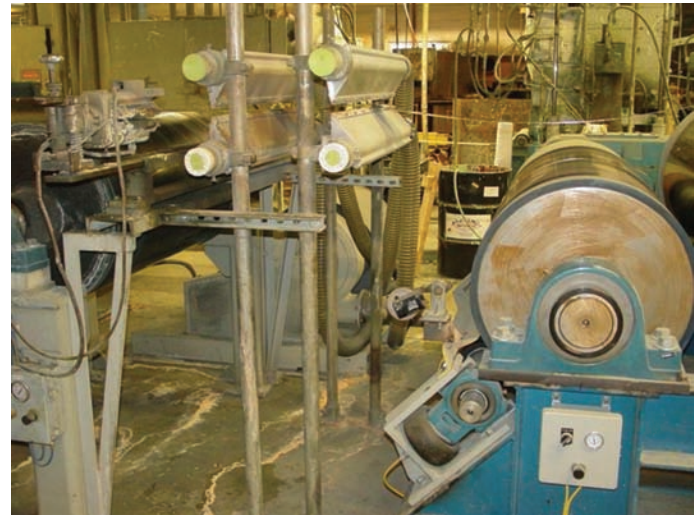
Air Knife installation with product web and blower installation.
